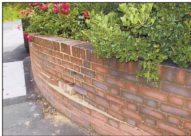
Damaged: James Hall's wall
